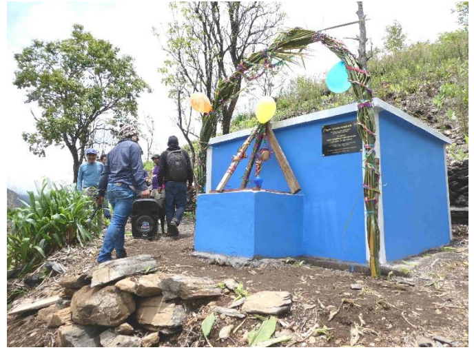
Stored in this main tank near to the agricultural areas are 9 cubic metres of water.
