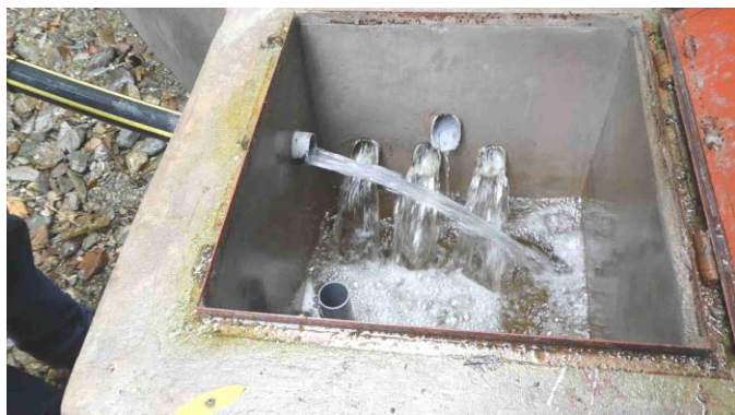
Close-up of the water chamber. There are three more of these to allow the water to flow to the main tank 3 km away.
